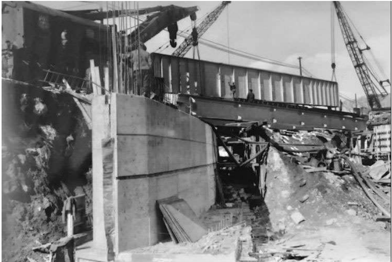
North Main Street during construction of the Underpass project to reduce grade level railroad crossings.
